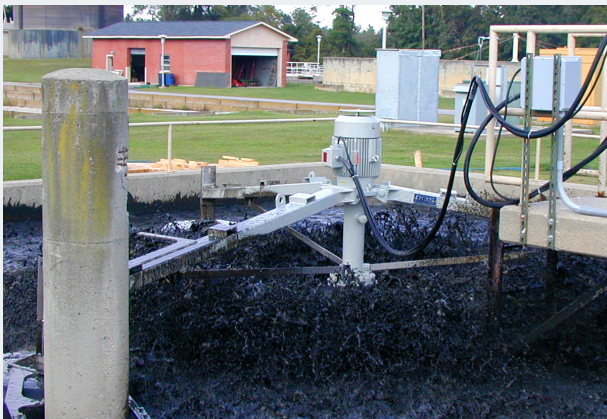
Post Mounted AERATOR
